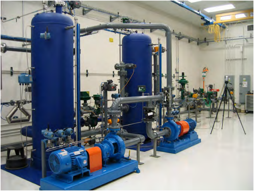
Figure 2.2 Performance Test Loop
